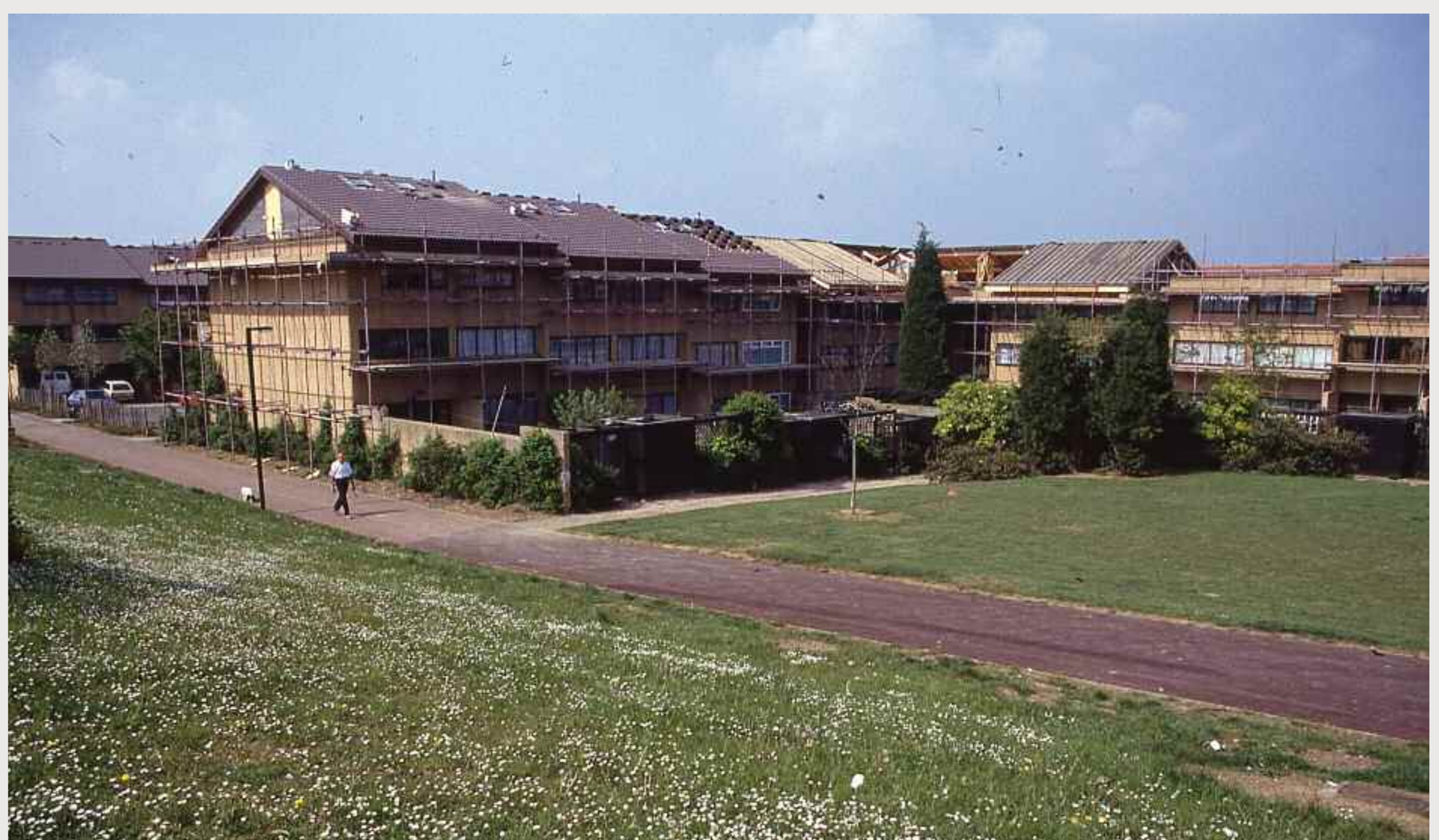
Reroofing of houses and flats in Conniburrow, scaffolding, man with dog on Redway bordered by white flowers. Image copyright of Homes & Communities Agency, courtesy of Milton Keynes City Discovery Centre.
