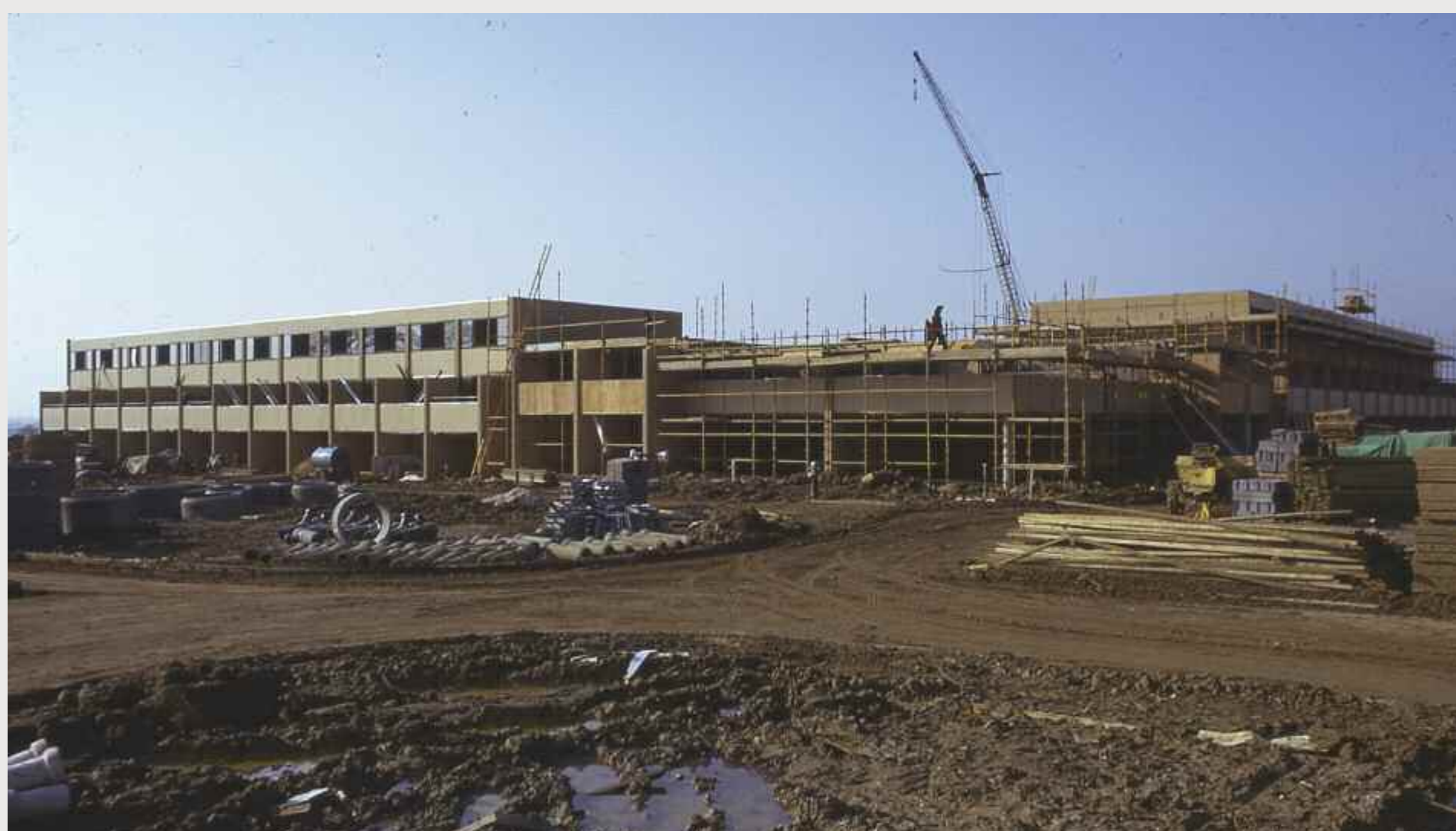
General view of housing under construction at Fishermead. Photograph by John Donat. Image copyright of Homes & Communities Agency, courtesy of Milton Keynes City Discovery Centre.
