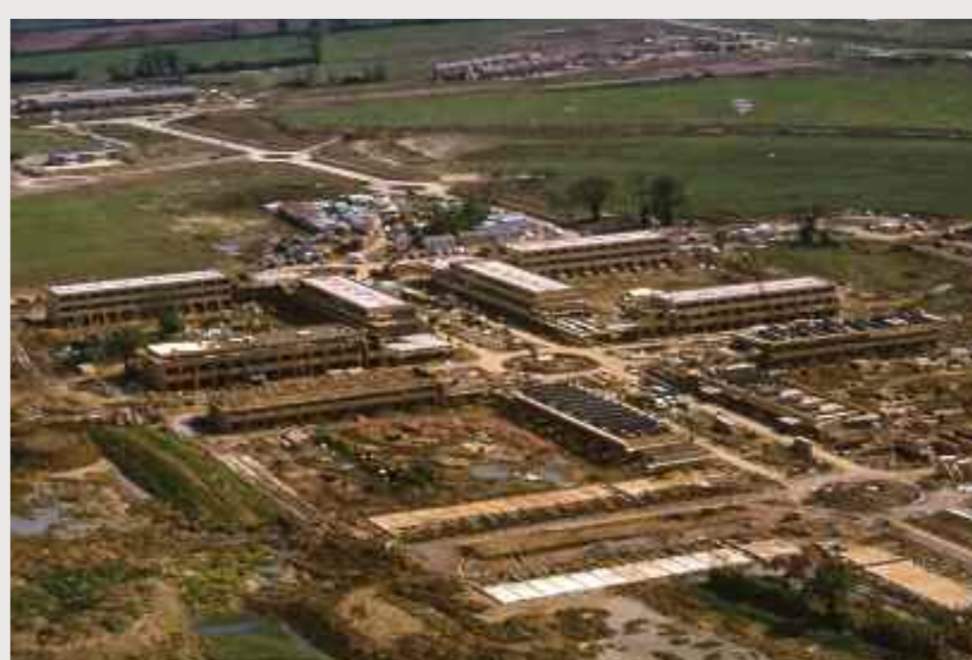
Aerial view of housing under construction at Fishermead, 1975. Photograph by John Donat. Image copyright of Homes & Communities Agency, courtesy of Milton Keynes City Discovery Centre.
